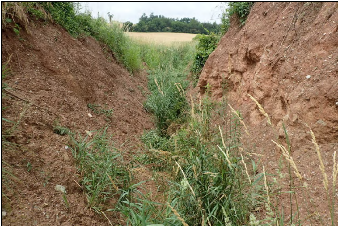
Appendix C2. Northwesterly view through the breach in the pond berm.
